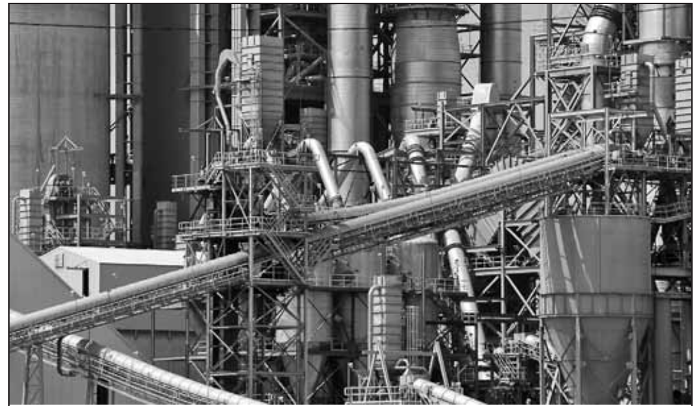
The revised standards affect facilities such as the Lehigh cement kiln in Maryland.
