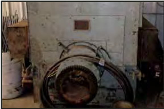
SIEMENS 1500 HP SHREDDER MOTOR 900 rpm, 3-phase, 4,000 volt.
