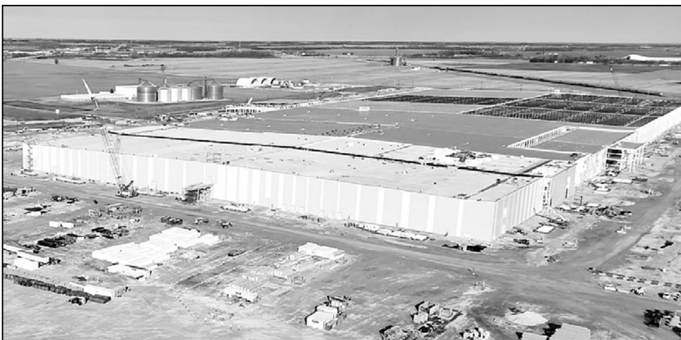
LG Energy Solution and Honda's two million square feet facility is expected to be completed by the end of 2024.
