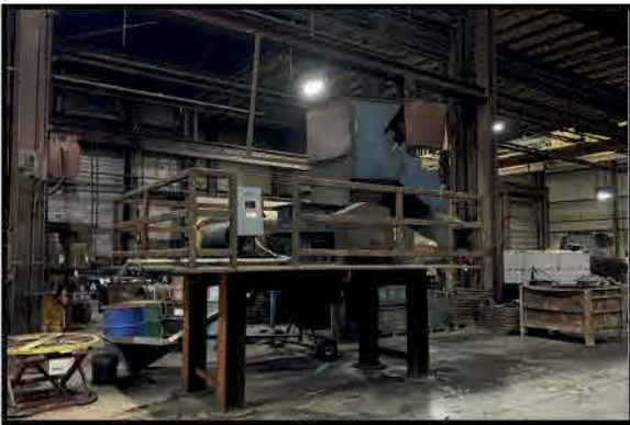
AMERICAN PULVERIZER WC-18 HAMMERMILL 30HP. 18" ROTOR. TAKEN OUT OF SERVICE A FEW YEARS AGO.
