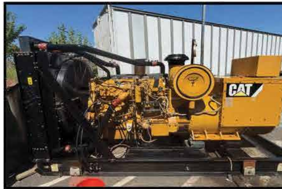
2008 CATERPILLAR 545 KW PRIME GENERATOR HOURS: 4,491, 3 PHASE, 480 VOLTS, 819 AMPS
