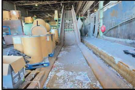
SINGLE STREAM RECYCLING SORTING SYSTEM LUBO SYSTEMS OCC SCREENER W/BOLLEGRAAF CONVEYANCE
